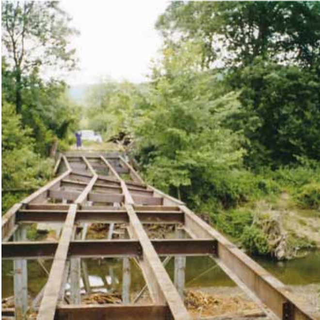
Reconstruction of the destroyed hydro-technical infrastructure and stream regulation near Karpacz. Photo: PARP archives
