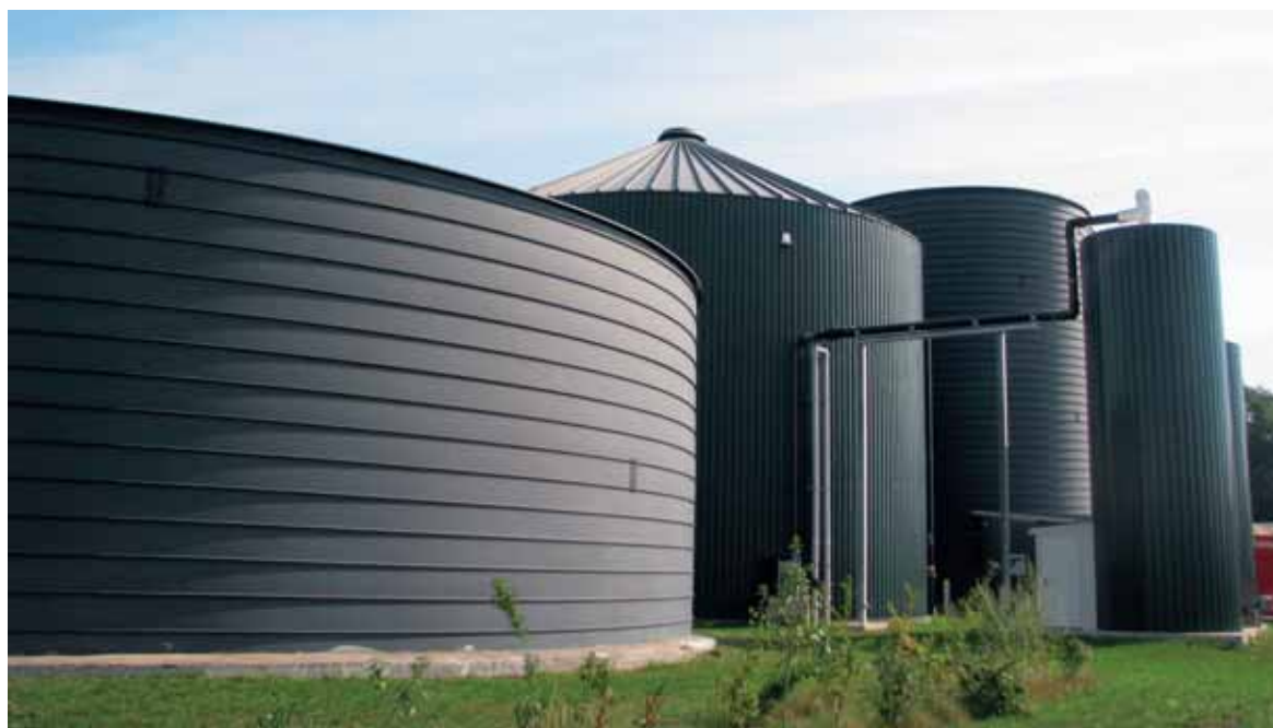
Local biomass heat plant
