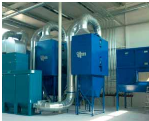
Low temperature system biomass drying systems – PWC hall
